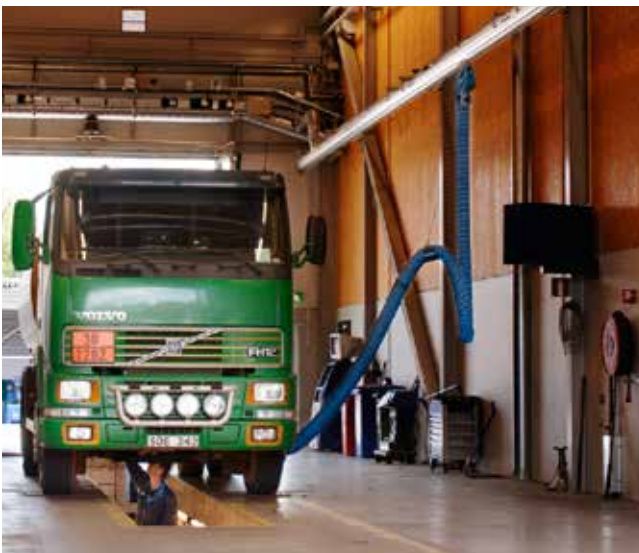
Example exhaust system for vehicle inspection.
